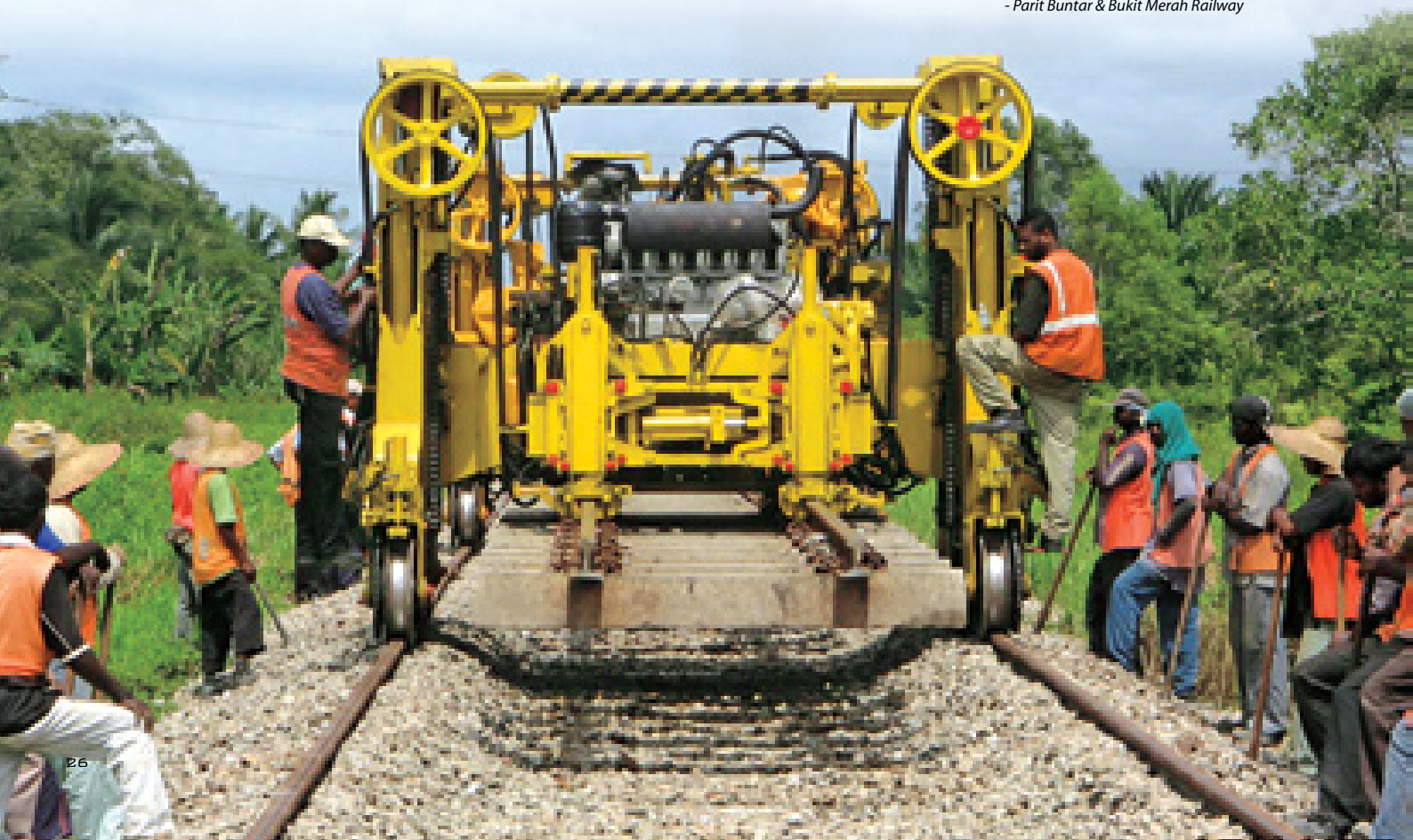
PQRS gantries picking up existing concrete sleeper panels - Parit Buntar & Bukit Merah Railway
